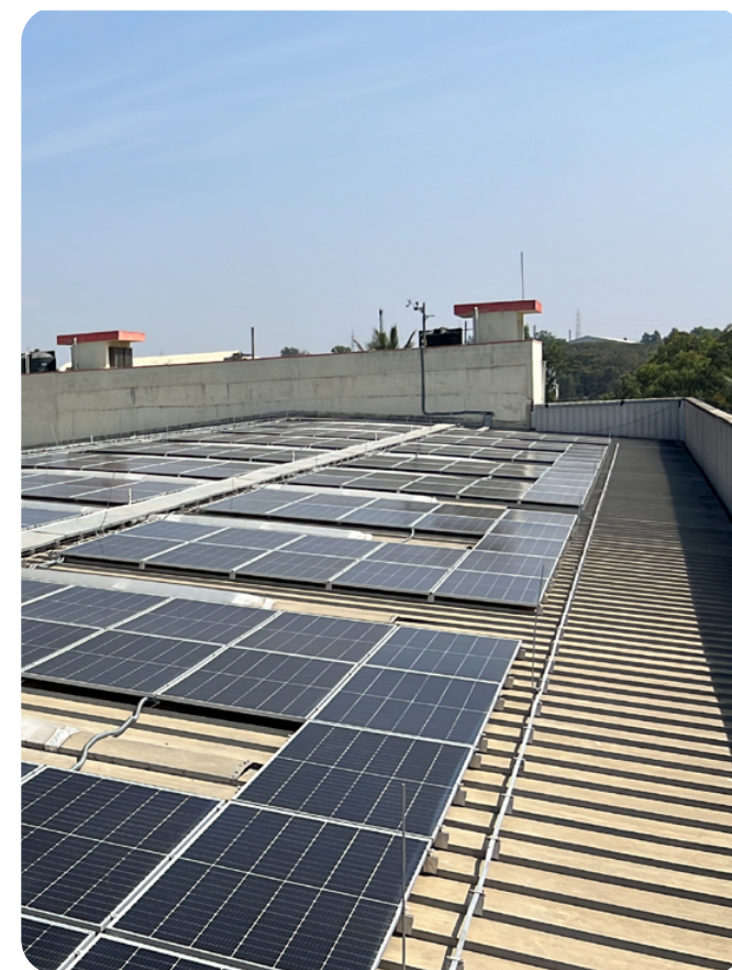
Solar roof at ITC Filtrona in India
