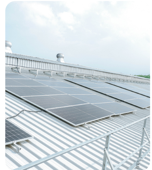
Solar roof installed at Filtrona Indonesia
