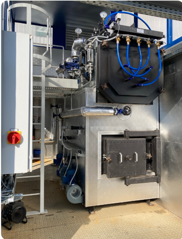
Biomass boiler at Filtrona Hungary
